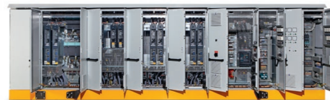
ELECTRICAL POWER DISTRIBUTION BOARD
